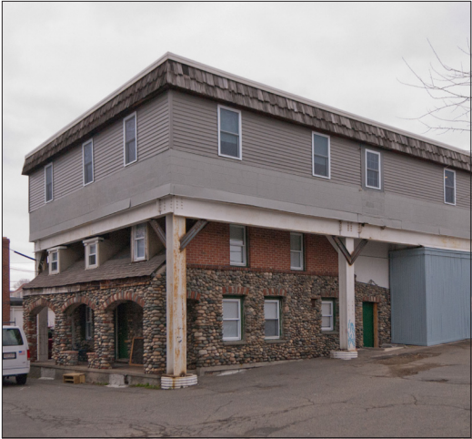
This 3rd floor addition overwhelms the historic building and is inappropriate. Its scale is substantially larger, the side gable roof form has been altered to a flat roof, the footprint has been greatly expanded, the window size and proportions is dramatically different, and trim, details and materials vary greatly from the historic building.
